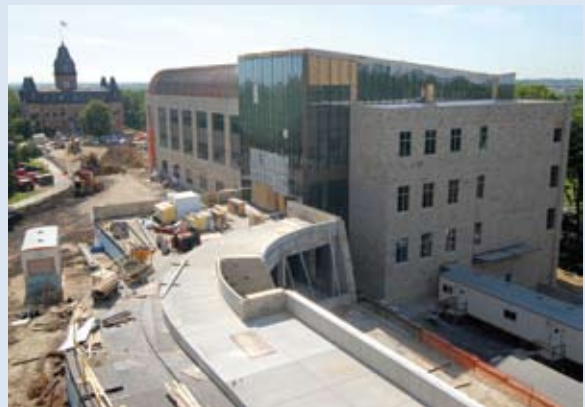
St. Olaf's new Regents Hall of Natural and Mathematical Sciences, a comprehensive teaching and research facility, is seeking LEED Platinum.
